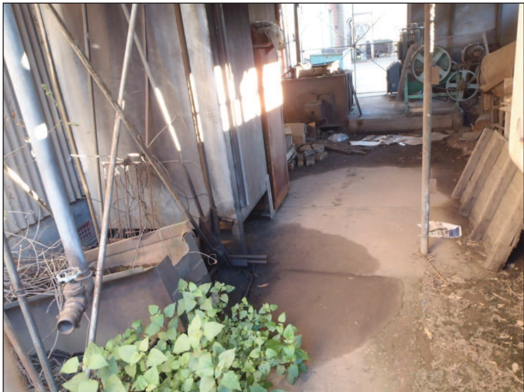
Plate 23 – Dark staining underneath AST 3 in Location 27.
