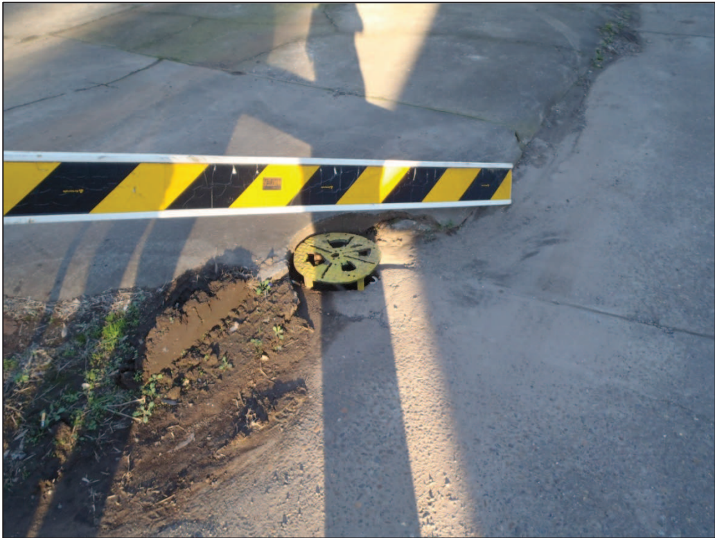
Plate 31 – Broken drain east of the Coils Factory.
